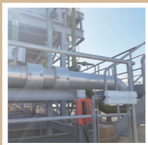
A Power Plant in Gibraltar
